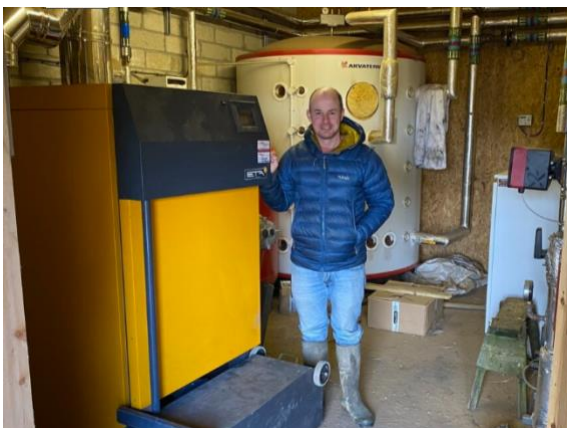
Mr. Andrews in the boiler room
